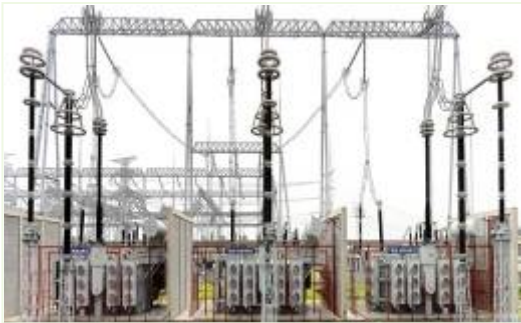
The world's largest 1000kV transformer
