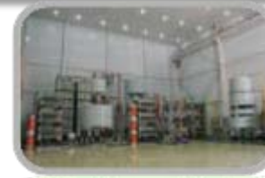
Flexible transmission technology sub-center
