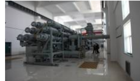
220kV smart substation in Xi'jing
