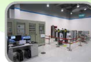
Smart power consumption technology sub-center
