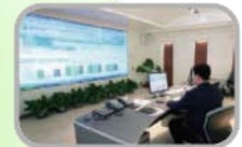
Information security technology sub-center
