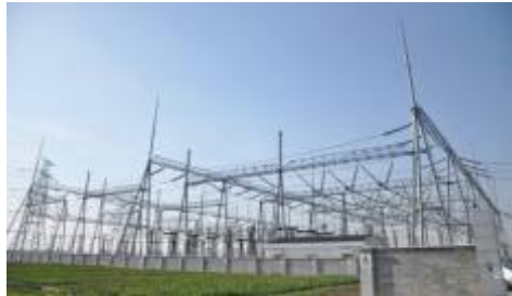
750kV smart substation in Yan'an
